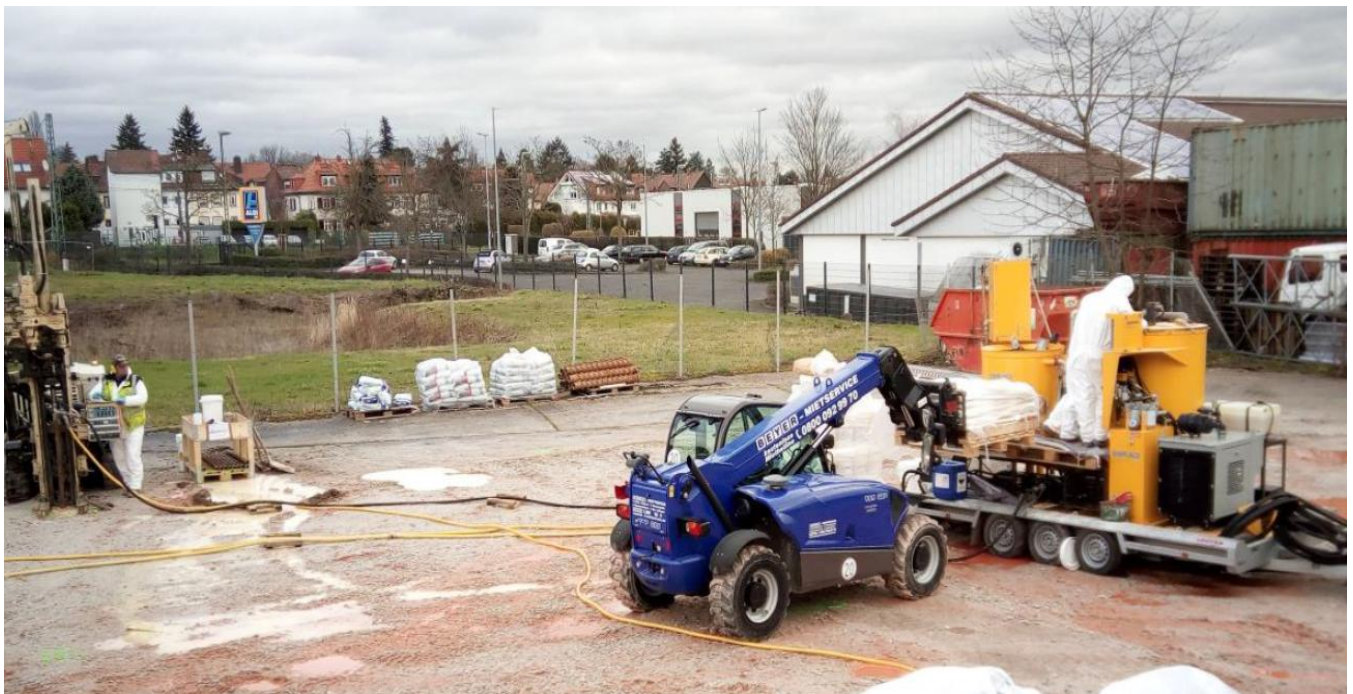
High pressure injection/fracturing/ and mixing equipment used for fracture-emplacment of persulfate-peroxide oxidant slurry into subsoils through direct push drill holes
