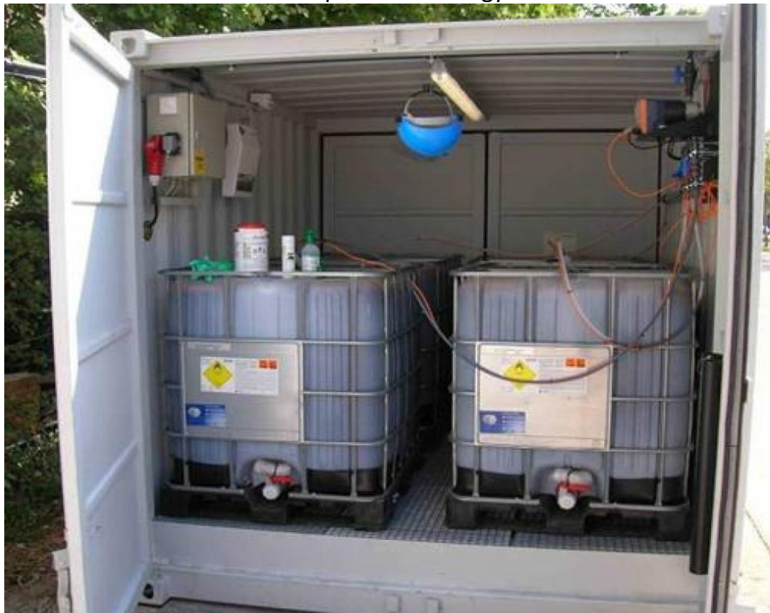
ISCO dosing station
