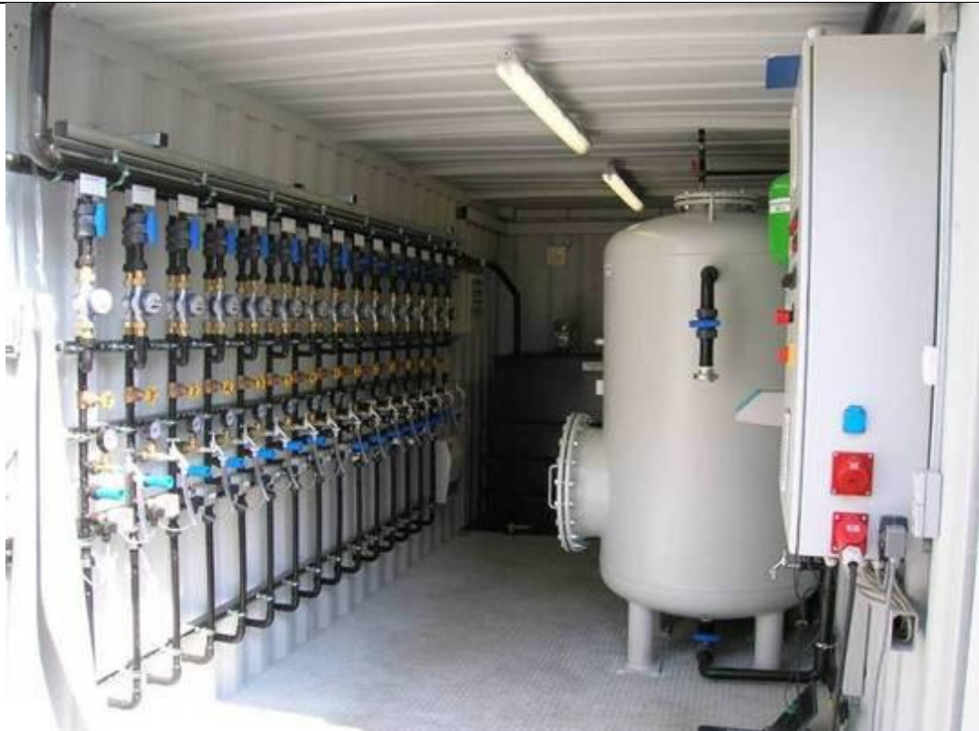
ISCO plant technology
