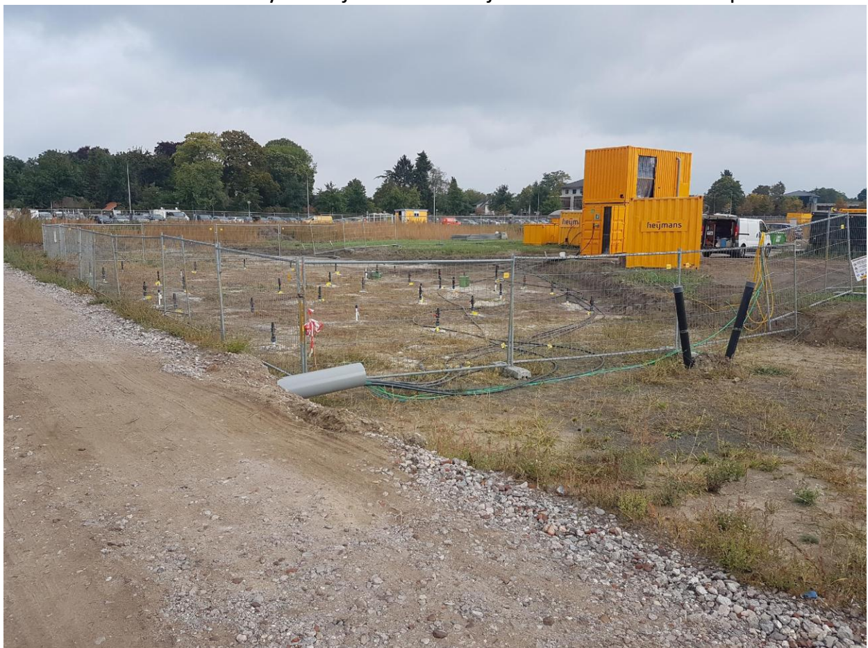
Overview injection filters in source zone
